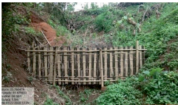
Brushwood Check Dam
